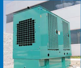
Back-up Generator Power
